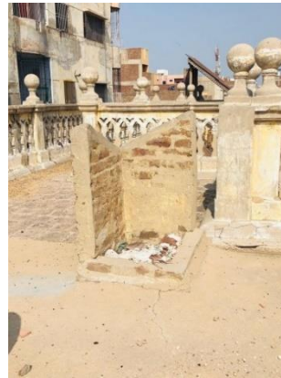
Fig 7: Damaged and closed wind catcher in an old building of Hirabad.
