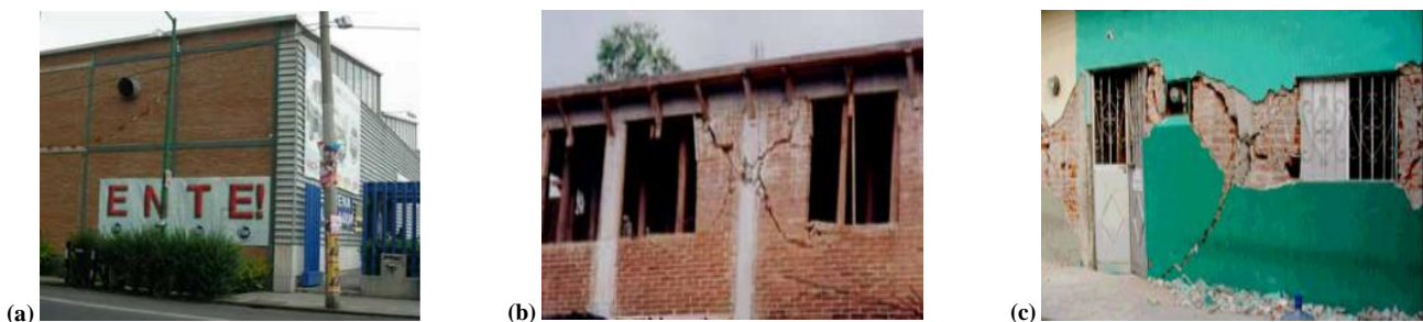
Fig. 5: Confined masonry construction in Mexico (a) an engineered structure in the industrial zone, (b) minor damage of confined masonry (c) major damage of confined masonry due to inadequate confining elements and their arrangement [34]
