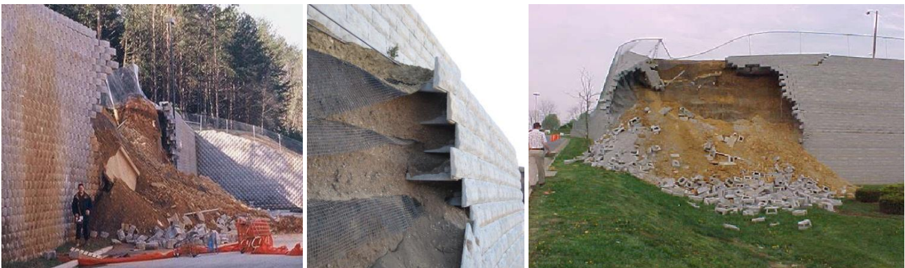
Fig 1: Failure of MSE wall.
