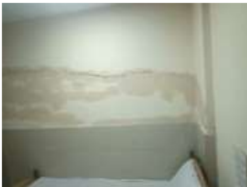
Figure 16: Hairline cracks due to water seepage in wards, Source; Author's fieldwork, 2019
