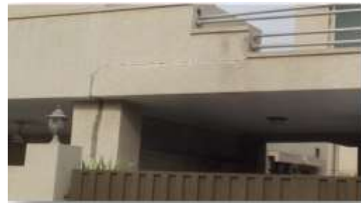
Fig. 5: Cracks On Parapet of Residential Building, Source; Author's Fieldwork 2019
