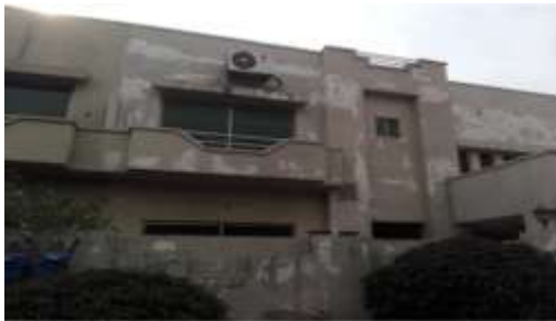
Fig. 4: External Finishes Peeling of a House under Survey, Source; Author's Fieldwork 2019
