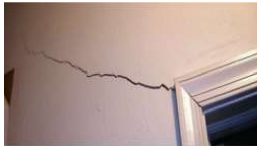
Fig. 6: Structural cracks on Walls of Residential Building, Source; Author's Fieldwork 2019
