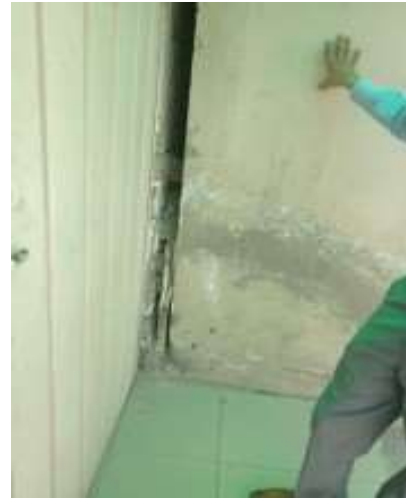
Figure 17: Water seepage in Expansion joints, Source; Author's fieldwork, 2019
