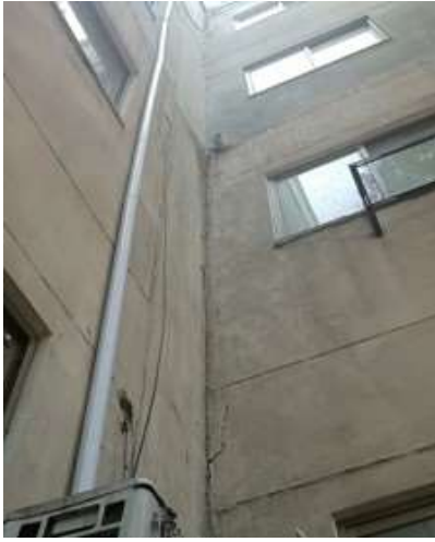
Figure 18: structural cracks on walls, Source; Author's fieldwork, 2019
