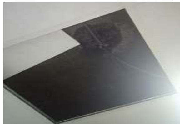
Figure 17: Sanitary fitting leakage above false ceiling, Source; Author's fieldwork, 2019
