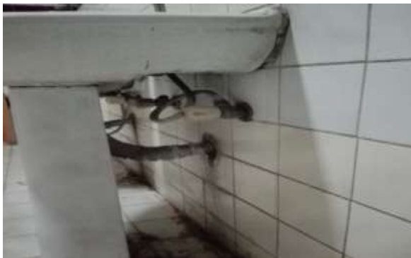
Figure 14: fungus growth and damaged sanitary fittings, Source; Author's Fieldwork 2019
