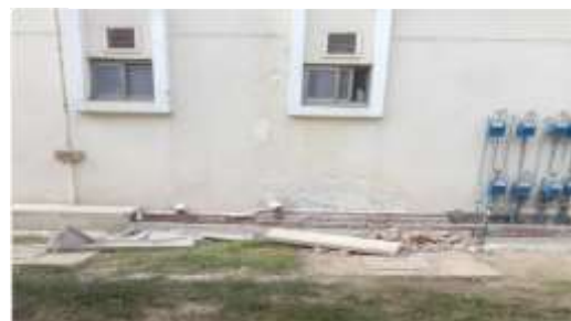
Fig.9: Damaged substructure of Apartment Building, Source; Author's Fieldwork 2019
